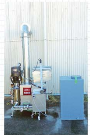
KESMAK KS-3 (specification of SUS316) Composting facility For processing alkali odors 30m 3 /min + Chemical injection system
