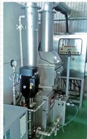
KESMAK KS-3 (specification of SUS316) Composting facility For processing acid odors 30m 3 /min + Chemical injection system
